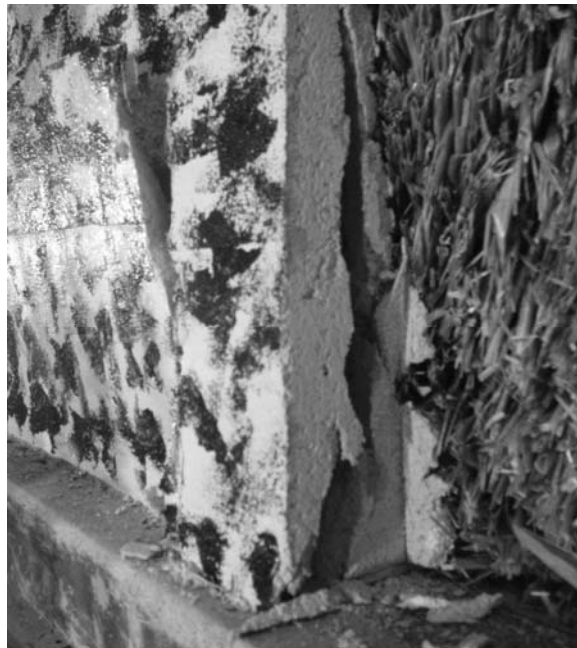
Figure 6.12b: Failure of Specimen E13
