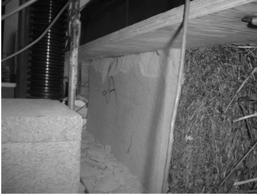
Figure 4.10: Bearing Failure of a Plastered Straw Bale
