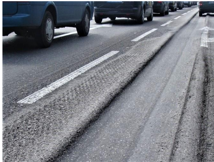
Figure 2.3: Rutting on asphalt pavement [23].
