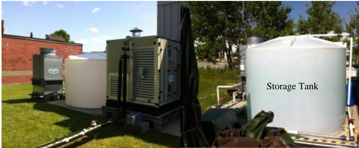
Fig. 3-6: 6000 liter CWS tank at Queen's University
