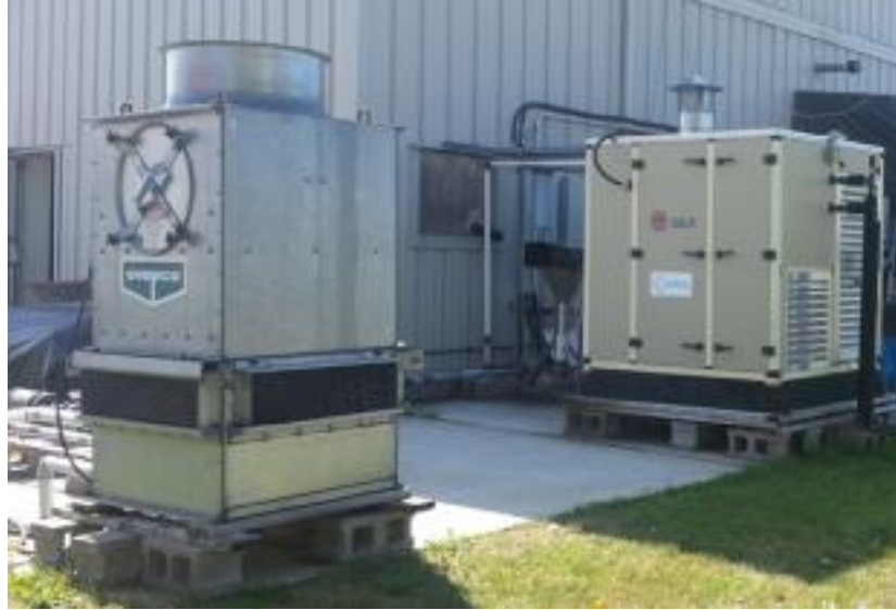
Fig. 2-5: Cooling water system at a commercial LDAC system at Queen’s University
